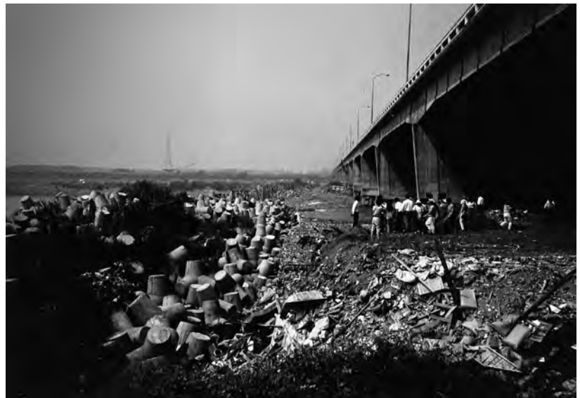
Figure 13. Undercutting and grade control efforts along the downstream side of the Kaoping Bridge over the Kaoping River, Taiwan, to control incision caused by massive gravel mining downstream. (Photograph by the author, October 1995.)
